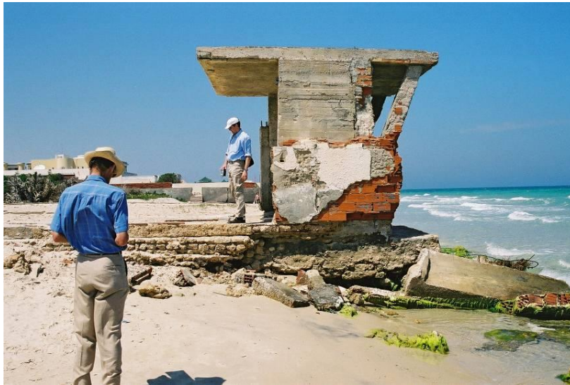
Figure 6. Beach erosion problem in Tunisia
